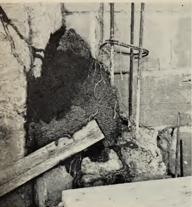
Fig. 13. Nest of a "tree termite," Nasutitermes corniger , on the wall of a building. Such nests are usually found in trees. Termites from this nest caused severe damage to another building 150 yards away. (Courtesy E. L. Moore.)
